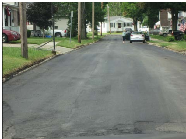
City crews began paving projects on June 12 in the area of 1st, 2nd and 3rd Avenues (above).
