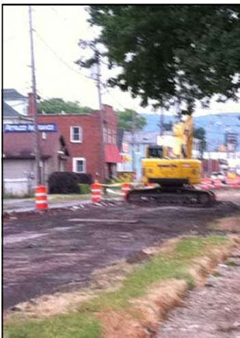
This "wide load" track excavator has an important job to do: bringing two-way traffic back to East State St.
