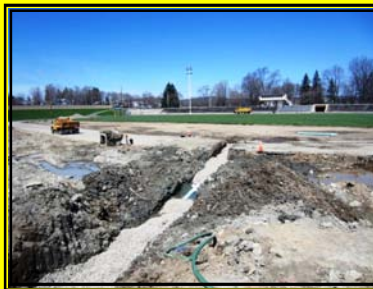
Bradner Stadium drainage work (above and left) will end decades of runoff impoundment (puddles) and extend the Stadium's useful season!
